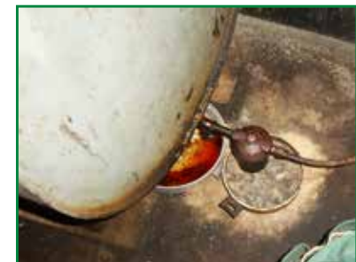
A leaking indoor tank
