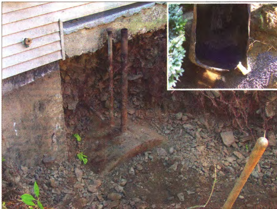
An abandoned underground oil tank. Inset photo: View of inside of open oil tank.
